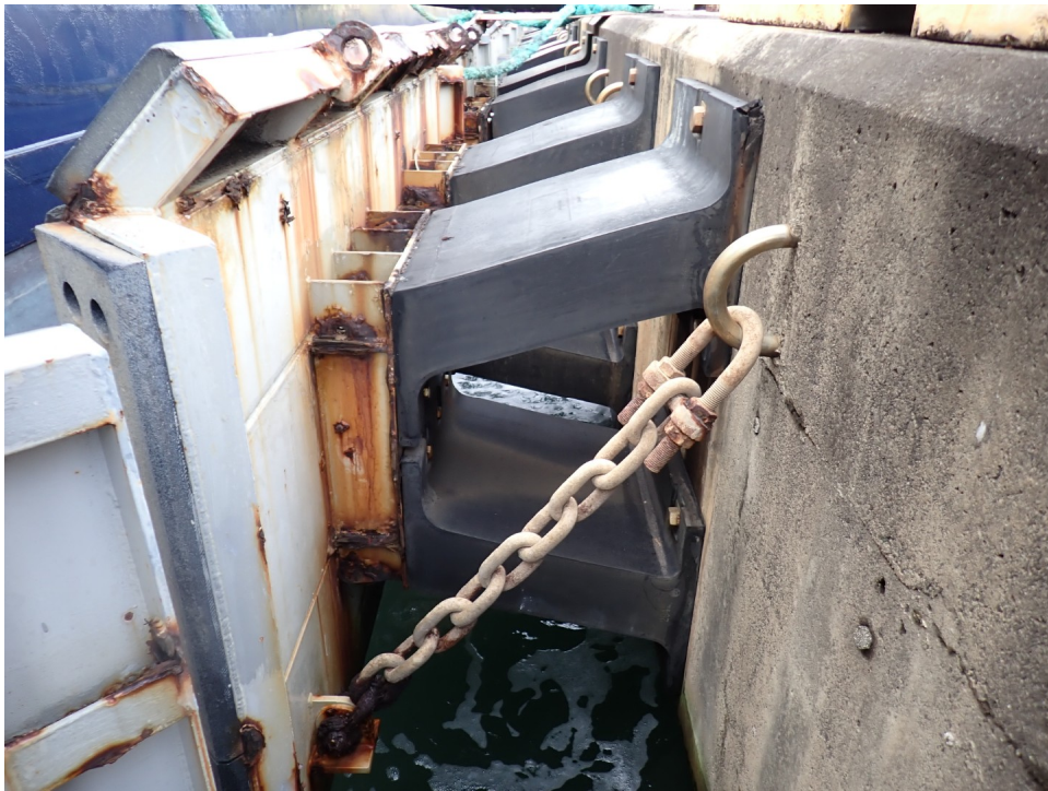
Photo 4: Existing Damaged Fenders
