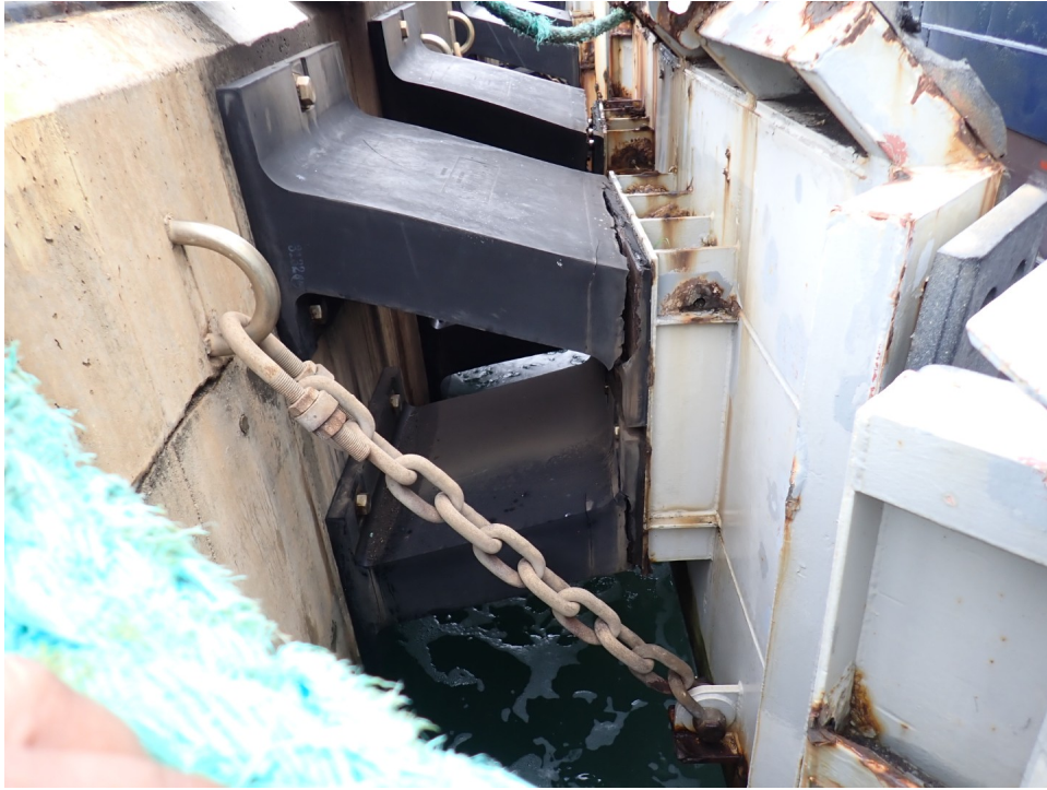
Photo 3: Existing Damaged Fenders
