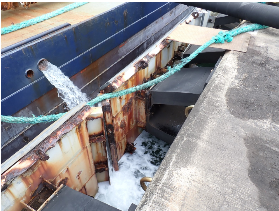
Photo 2: Existing Damaged Fenders
